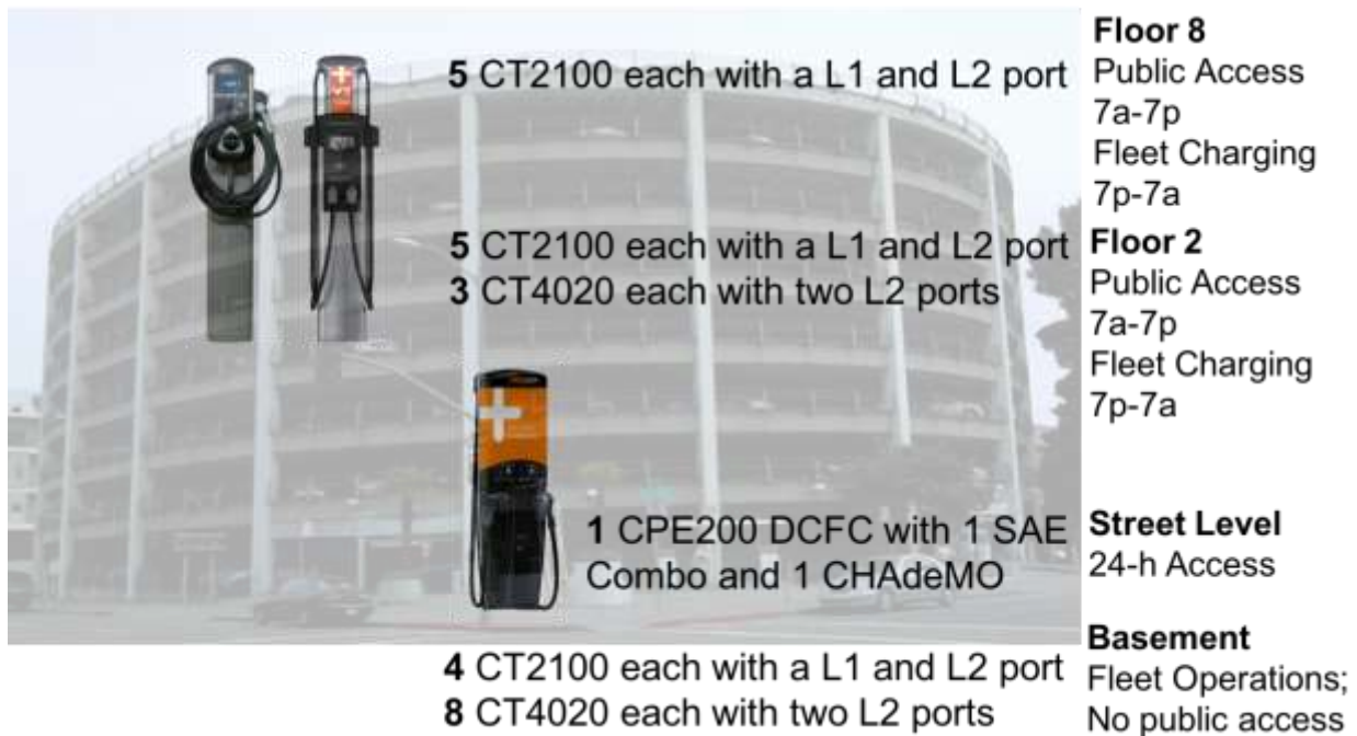
Figure 1: AlCoPark Garage Electric Vehicle Charging Stations
